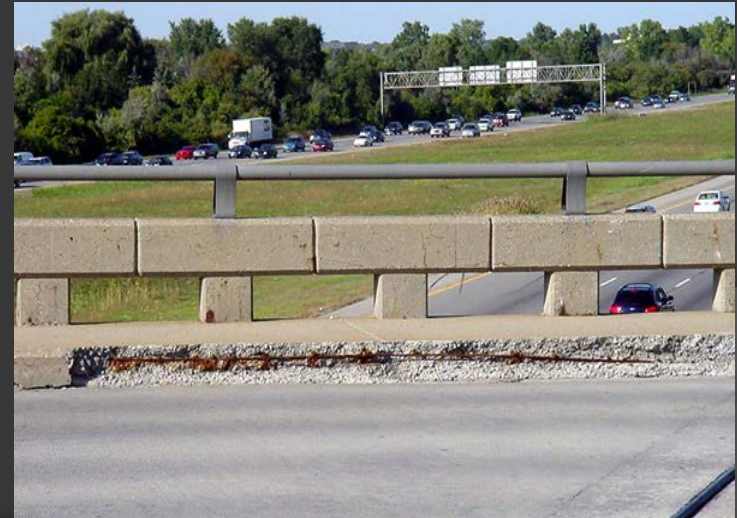
Crumbling Five Mile Road bridge over I-275 in Livonia
